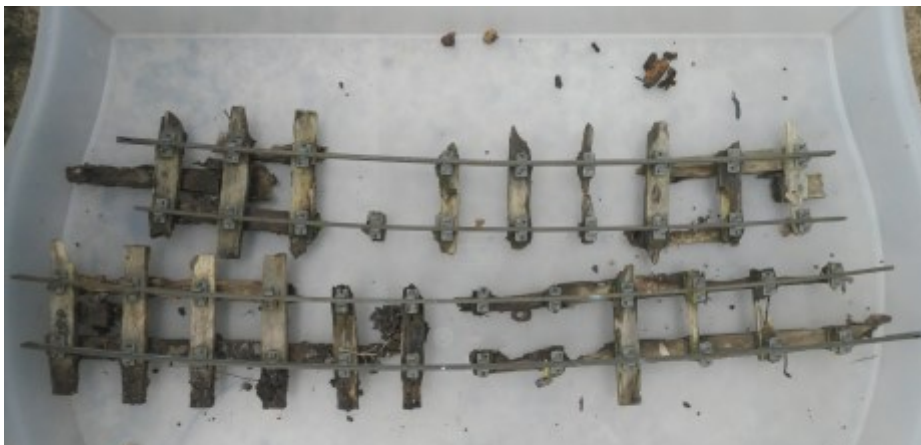
Photo 3 Serious rot of sleepers and battens.
