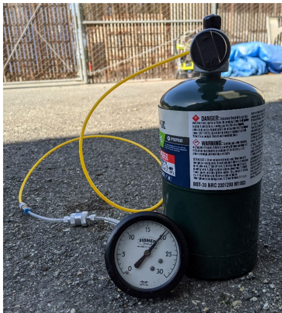
Figure 58. Measured pressure at highest valve setting 1.31 bar (19 psig)
