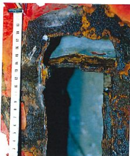
Figure 12.22 Failure at port side lug location at horizontal stringer.
