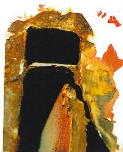
Figure 12.23 Failure at starboard side lug location at horizontal stringer.
