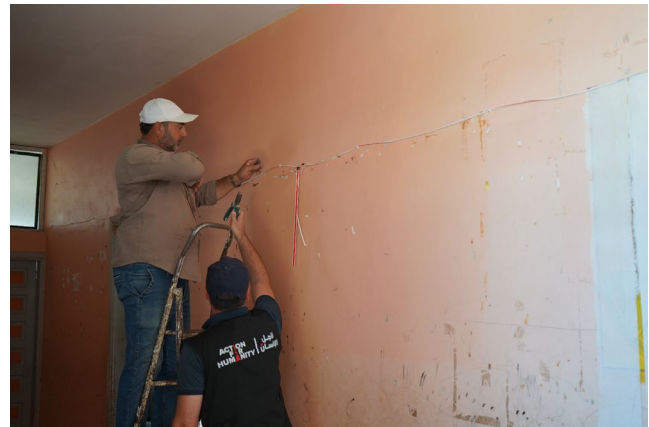
Installation of lighting in a school that hosts IDPs in Eastern Maliha in Dar'a Governorate. 25 July 2025. Photo Credit: © Action For Humanity NGO
