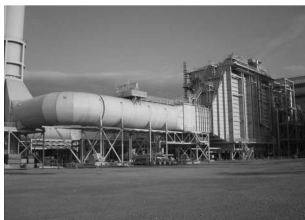
Figure 10 Group 4 stage 4-1 HRSG, exhaust duct
