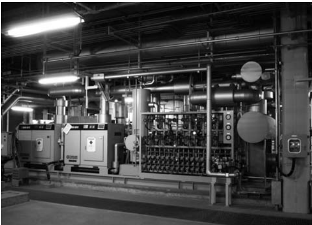
Figure 8 Clearance control system skid
