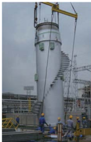
Fig. 18 Sample of Exhaust Stack
