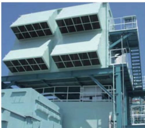
Fig. 11 Sample of GT intake filter house (1)
