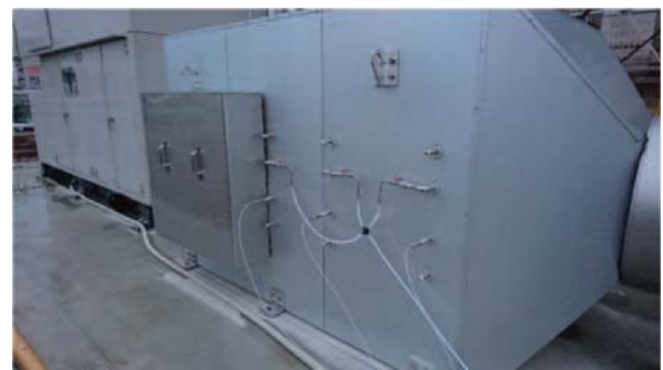
Fig. 6 NO x removal unit (SCR)
