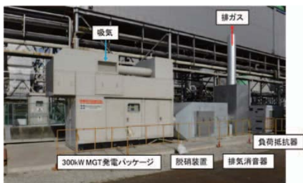
Fig. 1 300 kW ammonia combustion MGT package
