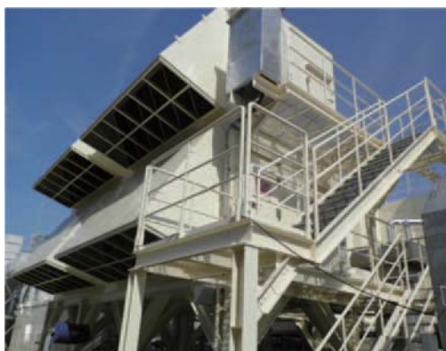
Fig. 12 Sample of GT intake filter house (2)
