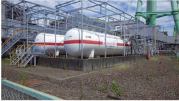
Fig. 4 Ammonia supply facility
