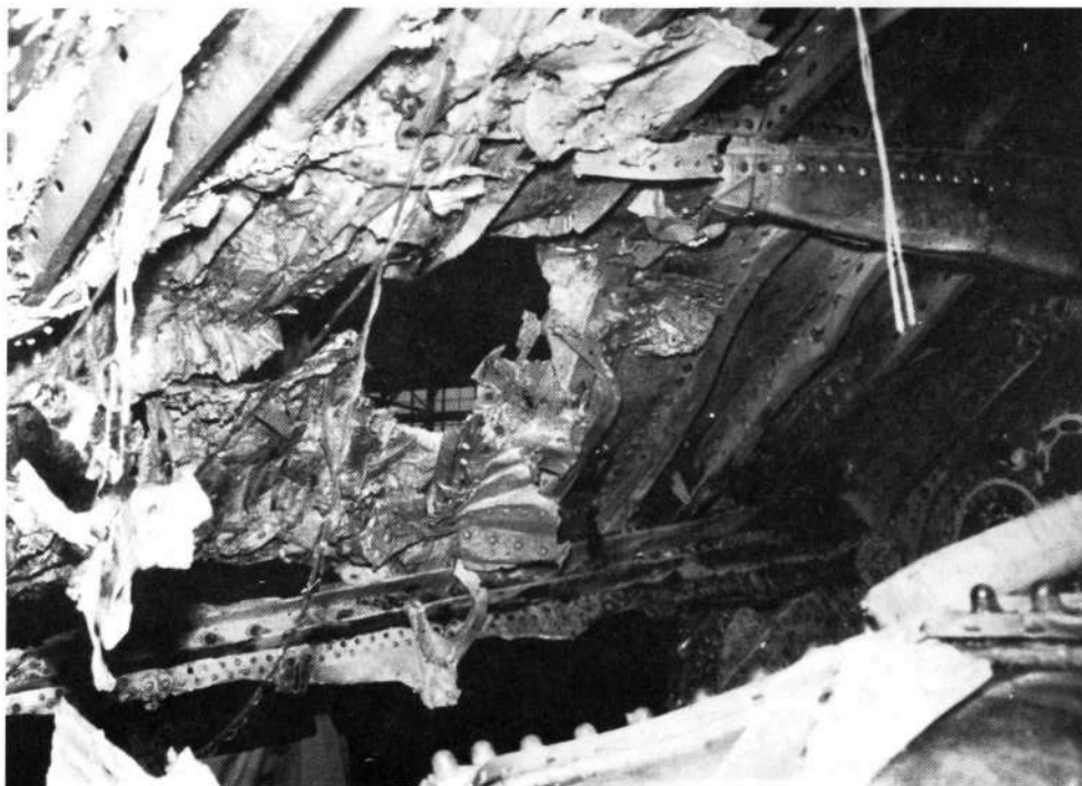
Figure DO12. Interior view showing extensive battering
