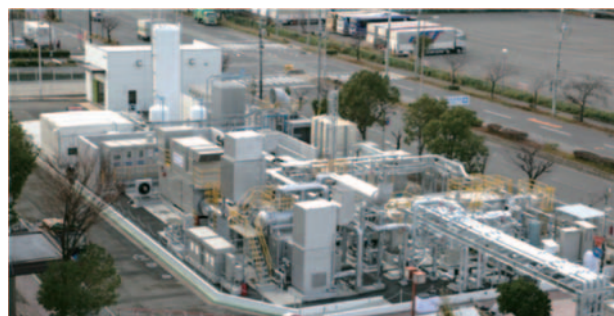
a) Hydrogen fueled power generation plant
