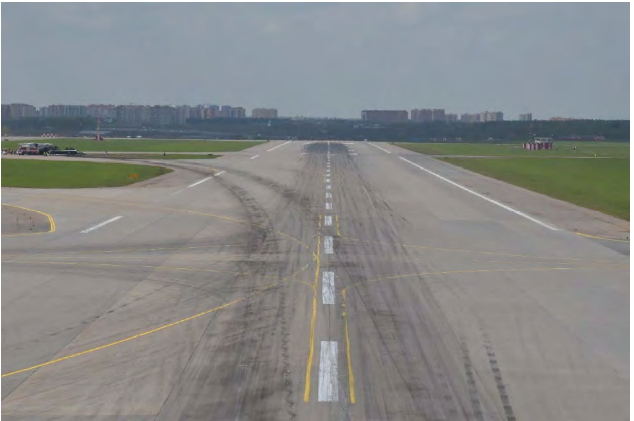
Fig. 39. The aircraft motion traces, the point of the RWY excursion at the area of the A3 TWY
