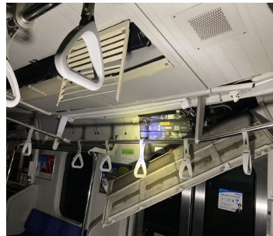
②先頭車客室損傷
