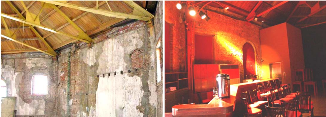
Figure 53 The restoration of the internal brick wall of the Octagon Building (Taken by the author).
