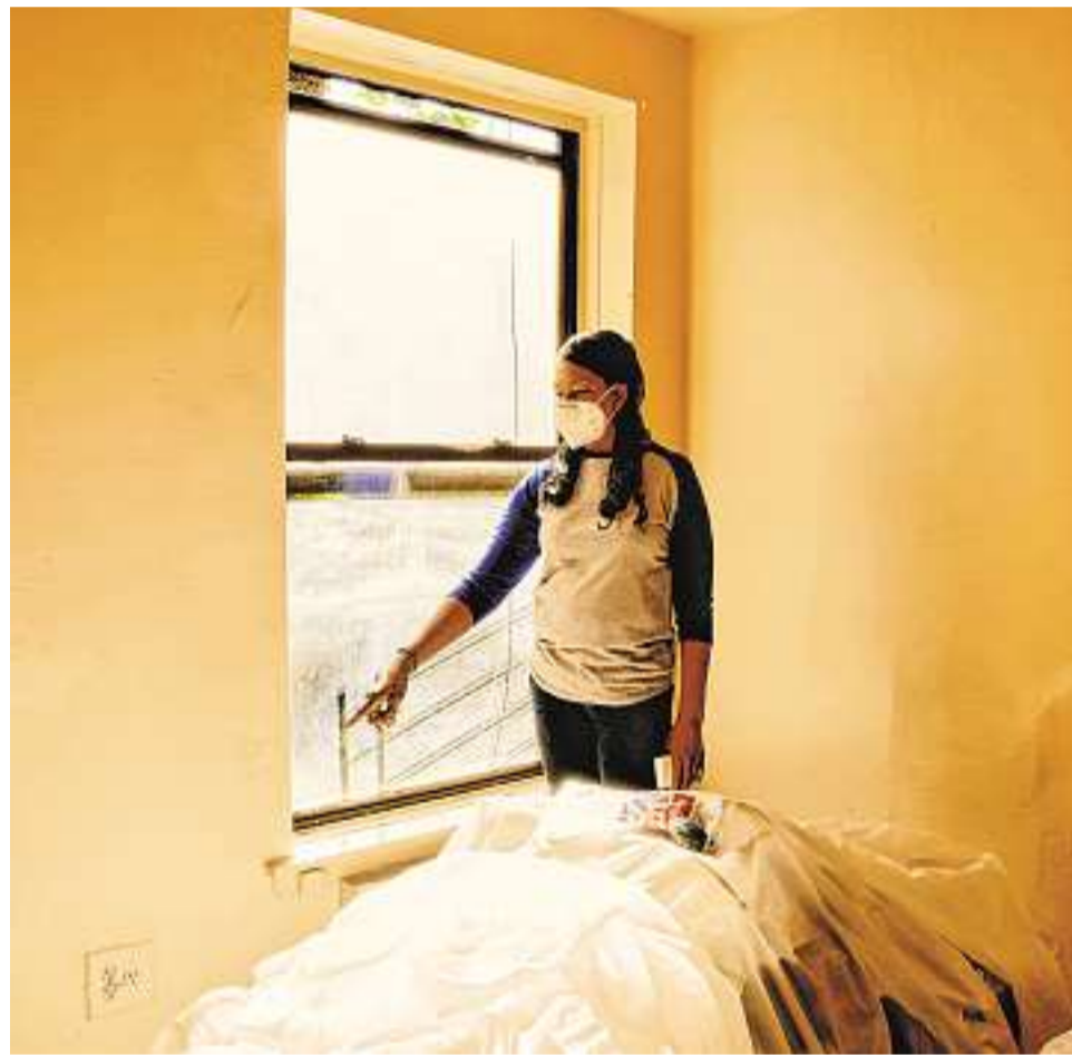
Mold in Cathy Stephens's apartment in New York was found to still be there after a paint job.
