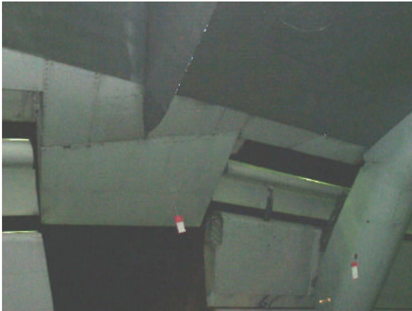
Figure A19. Damage on LH low speed aileron and flap track fairing - tagged debris
