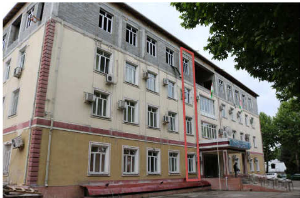
Photo 3: Front view of the main building of MOLME, by red shown the area where the elevator proposed to be mounted.
