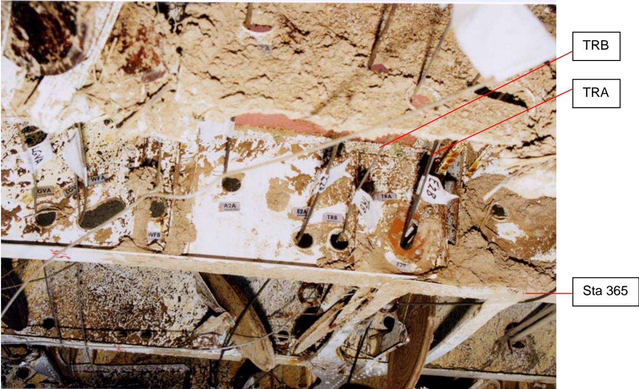
Figure 28.1 – No 2 Powerplant Cables Underfloor
