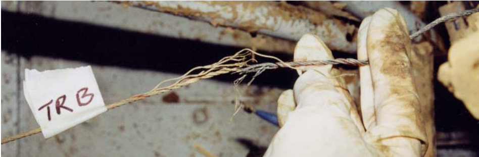
Figure 28.3 – Cable TRB Severance
