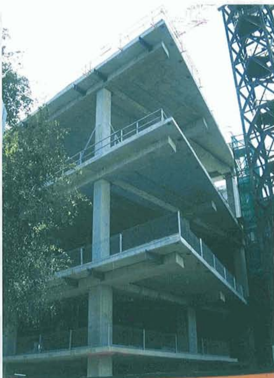
The re-development of Melbourne's GPO. Precast balcony units cantilever in two directions.
