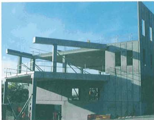
The precast skeletal frame of this four level office development was constructed in just 26 days.
