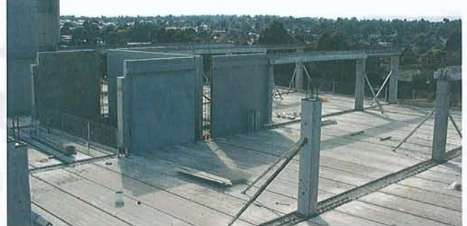
Precast components installed in an office project at the Tally Ho Business Park.
