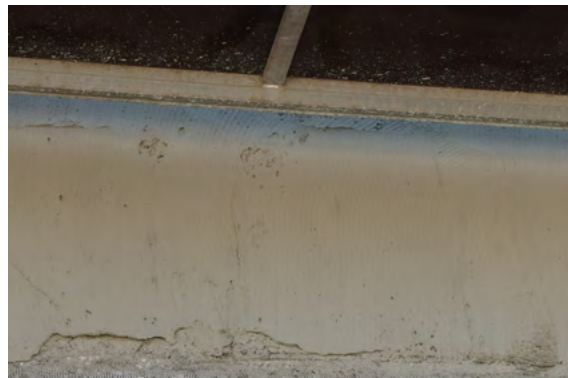
Application of a render, modified with SITREN AirVoid® 651 to an exterior facade
