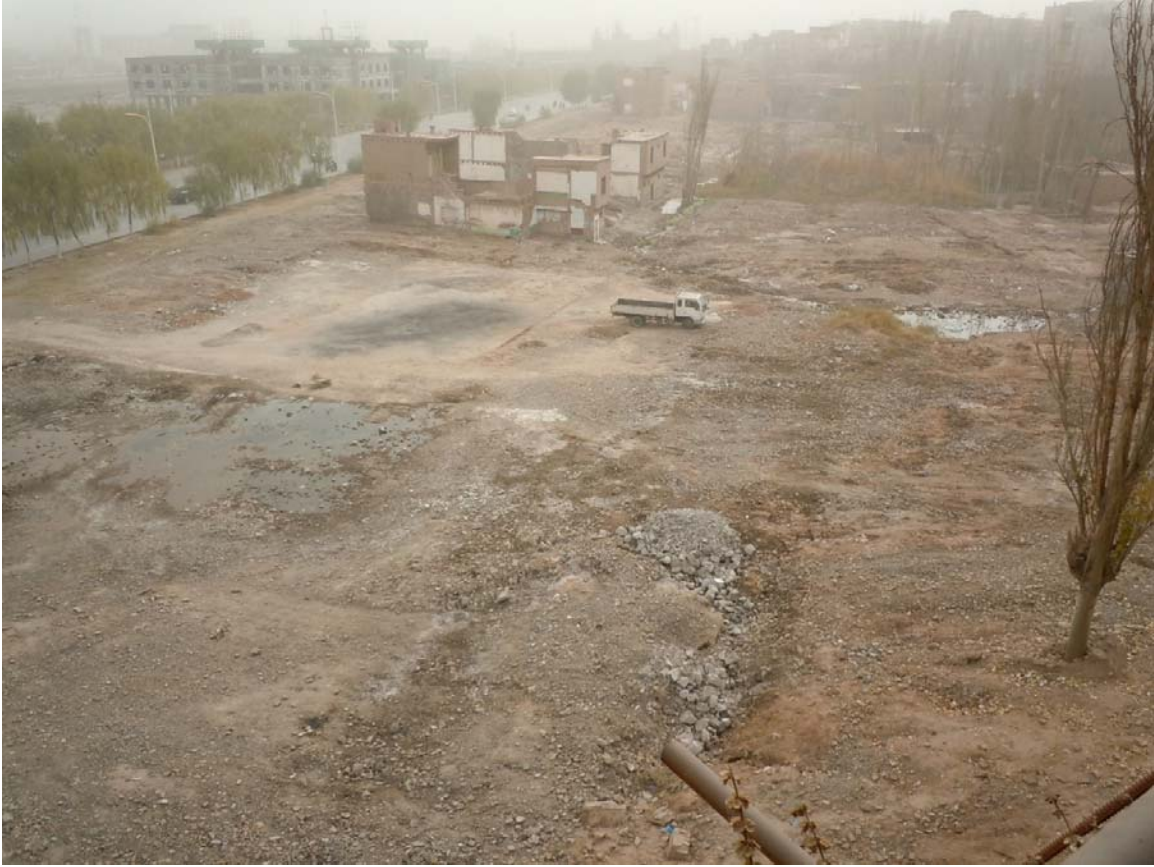
Photo 2. Homes removed east of northeast section.
