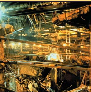
Photo depicting World Trade Center damage after the bombing in 1993.
