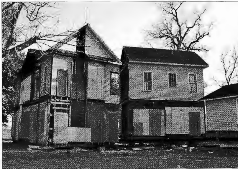
In order to move the Dew Plantation House to its new home, Historic Houston first removed parts of the structures that were not original to the house. Next, the house was cut into two pieces to facilitate the difficult move. Historic Houston, a non-profit organization, has had over 35 houses donated to them for relocation purposes since its founding in 1998.
