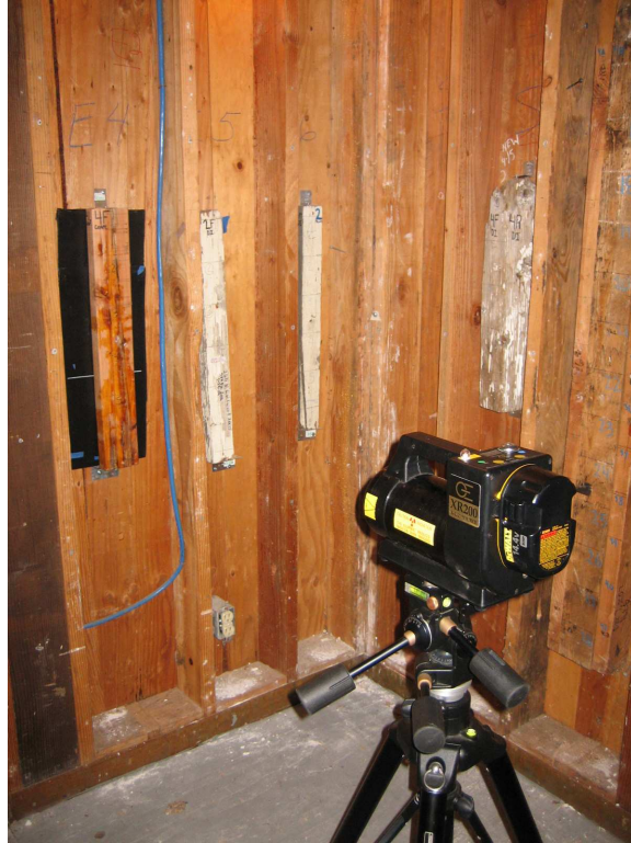
Figure 6. Test boards, imaging plates (in black cover behind far left board) and portal X-ray detection device used for field study. Test site, Villa Termiti Richmond, CA. The black device in the center of the image is a XR200 X-ray emitter (Golden Engineering, Inc., Centerville, IN).
