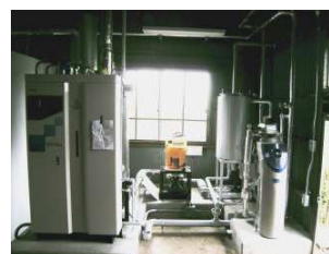
蒸気ボイラ (LPG)
