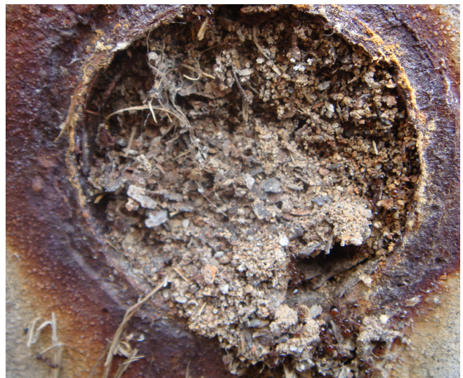
Fire ant nest inside of drainage pipe; Richmond, Va.
