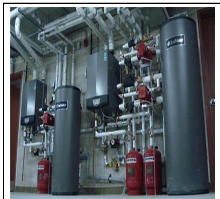
The MSFC Steam Distribution System is the second of a two phase project to convert buildings to a more efficient natural gas fired boiler system that reduces operating and maintenance costs.
