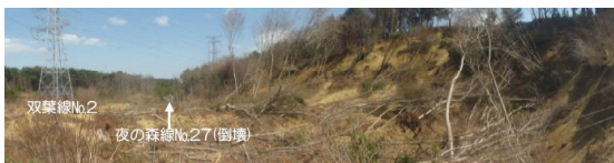
Overview of landslide
